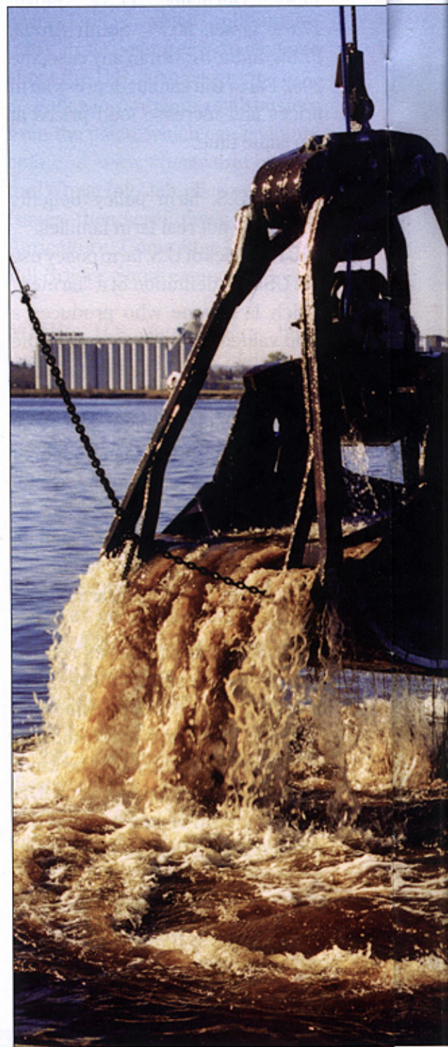
Pretty it isn't. But a program of responsible continuing dredging is vital to the success in the Twin Ports — and around the world.
