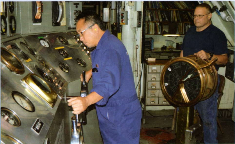
First Assistant Engineer Yvar Yap at controls. Qualified Member of the Engine Department (QMED) Tom Acton alongside the chadburn.
