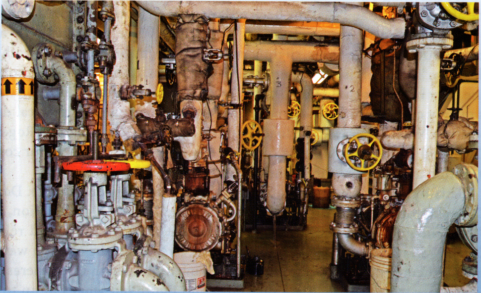
View of the engine room floor showing circulation pumps, feed pumps, water strainers and more. This room is a learning experience: everything you run into made of steel is going to hurt.
